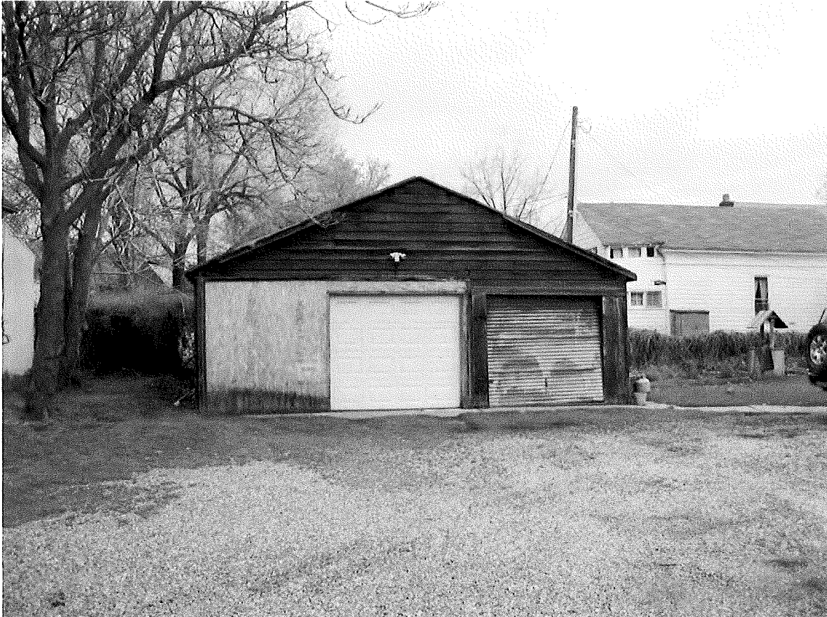
Figure 4: Circa 1950 three car garage (now converted to two car) that has deteriorated to the point that it must be removed.
