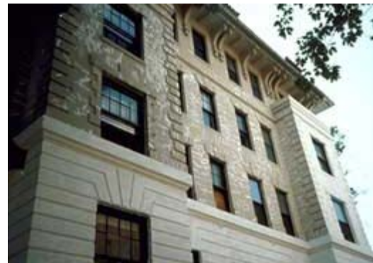
Caulking is not an appropriate method for repairing cracks in historic stucco. Photo: NPS files.
