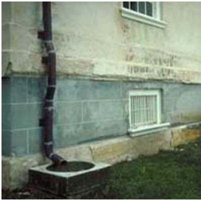
The damage to this stucco appears to be caused by moisture infiltration. Photo: NPS files.
