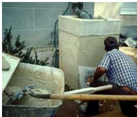
The deteriorated surface of this catch basin is being re-stuccoed. Photo: NPS files.
