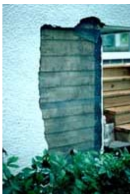
The stucco will be applied to the wire lath laid over the area to be patched. Photo: NPS files.
