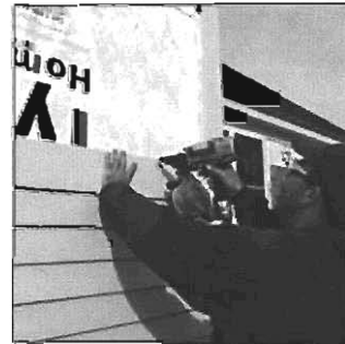
Engineered wood siding is cut and installed like hardboard, with a nailgun.
