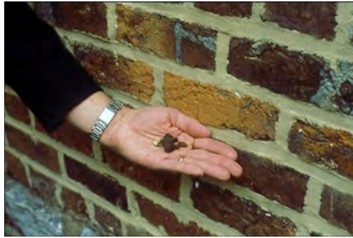
...which may lead to cracking, spalling.
