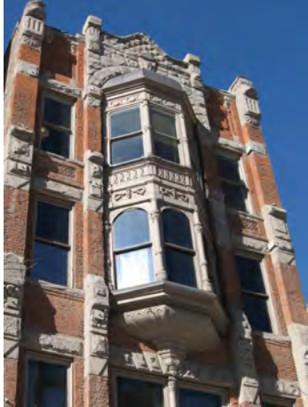
A combination of brick and decorative stone are featured on the upper facade of Daft Block, 128 South Main Street.
