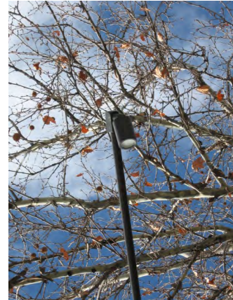
Above is an example of an appropriate exterior pole light (1136 E 3rd Avenue).
