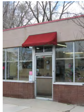
Simple shed roof canvas awnings are also appropriate for entrances such as at 442 N 300 West.
