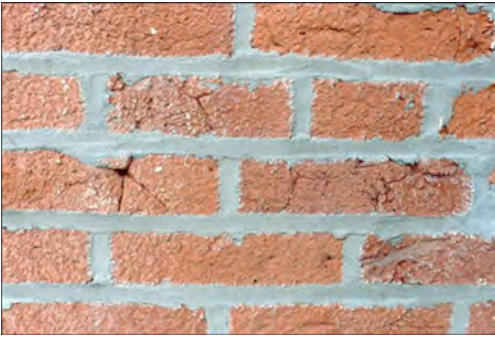
Hard mortars may force moisture through the more permeable brick and force mechanical stresses to be relieved through the softer brick...
