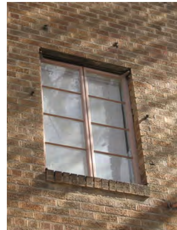
Original steel casement window at 702 E "K" Street. This window is significant to the design and character of the building.
