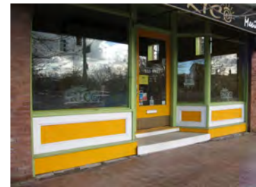
Original storefronts, such as those at 802 S 600 East (top) and 779 S 500 East (bottom), should be preserved and maintained.
