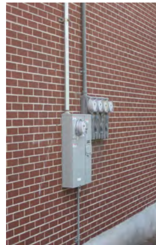
Meters at 39 N 'I' Street are correctly placed on a non-primary elevation.
