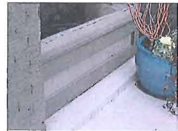
This rebuilt bulkhead at 361 N Center Street is a good example of in kind replacement.
