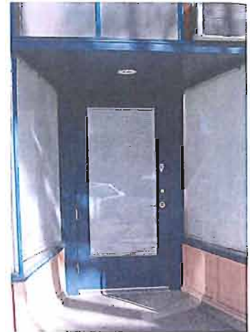
Rebuilt doors, such as this example at 428 W 300 South, should replicate the original as closely as possible.
