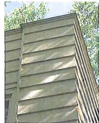
Original wood siding should be preserved and maintained. (801 E 1st Avenue).
