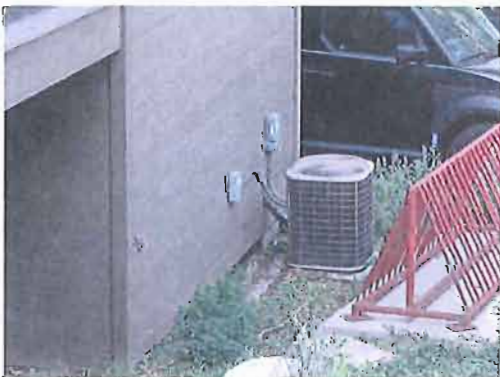
This HVAC system at 271 N Center Street is situated in an inconspicuous area on the rear elevation.
