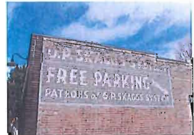
Historic "ghost" signs such as this one at 422-426 N 300 West should be preserved and maintained, not painted over.
