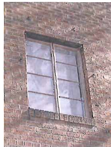
Original steel casement window at 702 E 'K' Street. This window is significant to the design and character of the building.
