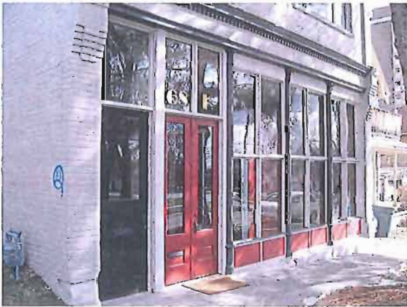
Good examples of rebuilt storefronts are those at 68 N 'K' Street (above) and 740 E 2nd Avenue (right).
