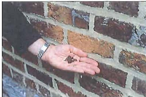
...which may lead to cracking, spalling and erosion..
