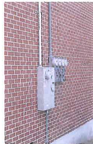
Meters at 39 N 'I' Street are correctly placed on a non-primary elevation.
