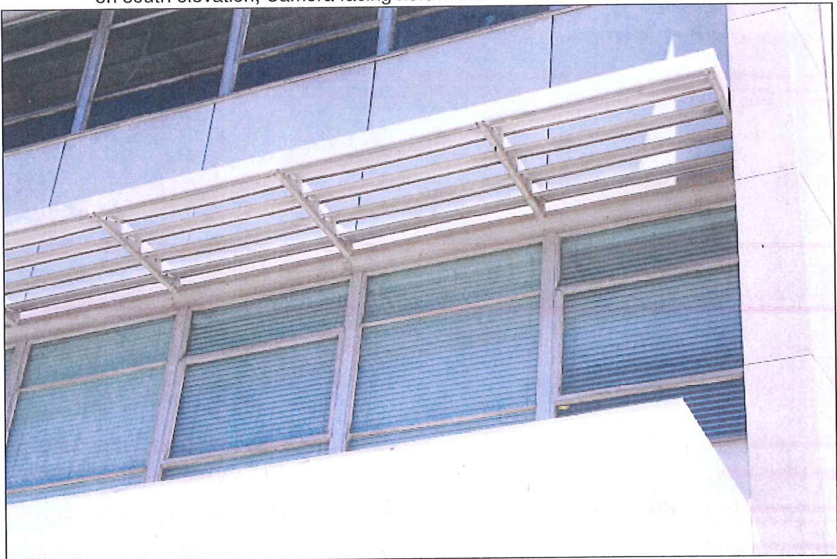
20 of 20. Pacific Northwest Pipeline Building; Close-up of aluminum louver window awning and window detail on south elevation; Camera facing north.
