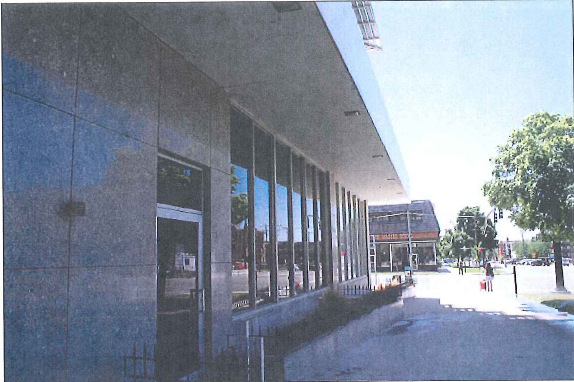
13 of 20. Pacific Northwest Pipeline Building; First (at-grade) story, west elevation window, projecting panel, and thin stone veneer detail; Camera facing south.
