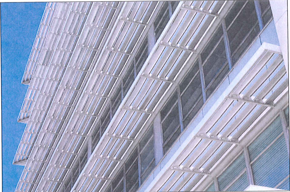
19 of 20. Pacific Northwest Pipeline Building; Overview of aluminum louver window awnings on south elevation; Camera facing northwest.
