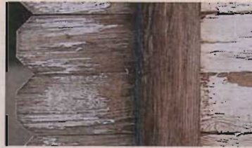
Wood rails and can require a great deal of maintenance.
