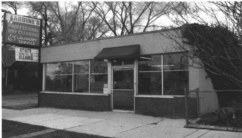
Many neighborhood commercial buildings were built with poured concrete pavement extending the width of the storefront. This example is at 442 North 300 West.
