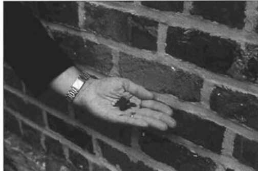
which leads to cracking and spalling.
