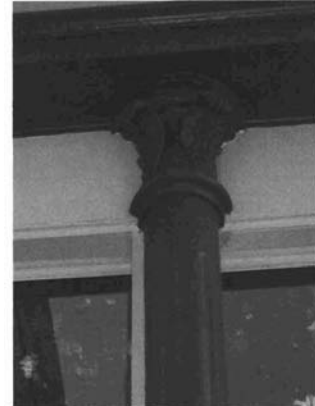
Cast iron details add to the historic character of a building (68 North K Street).
