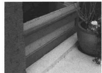
This rebuilt bulkhead at 361 North Center Street is a good example of in kind replacement.
