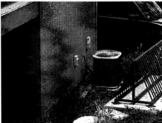
This HVAC system at 271 Center Street is situated in an inconspicuous area on the rear elevation.
