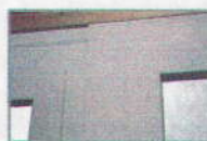
Closeup of interlock on wide rail door.
