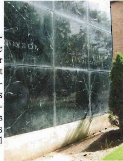
Marble paneled veneer on the main façade at 641-645 E. South Temple which was built in 1957.
