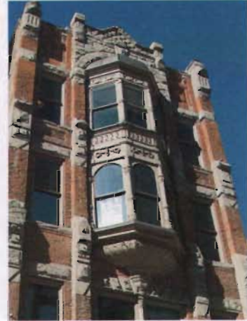
A combination of brick and decorative stone are featured on the upper façade of 28 South Main Street.
