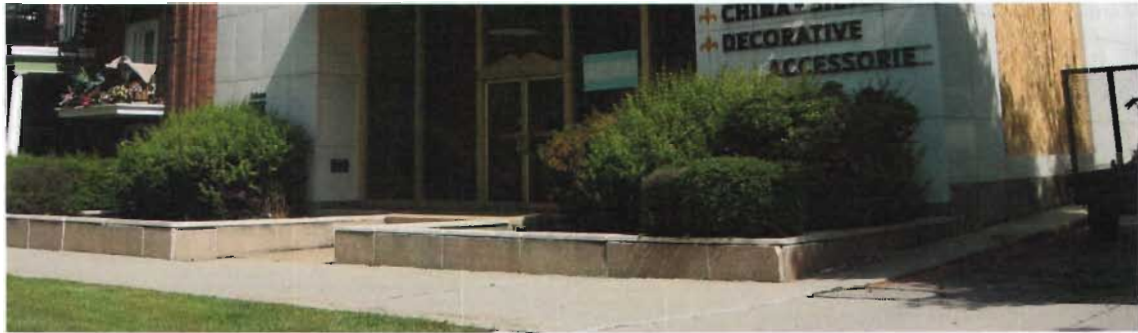
Masonry retaining walls in front of commercial buildings should be preserved and maintained such as this example at 445 E. South Temple Street.
