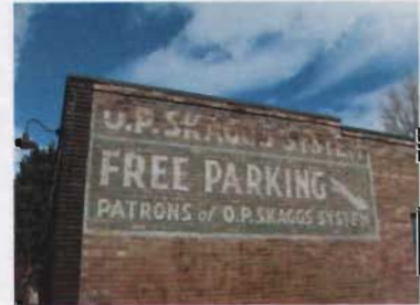
"Ghost" signs such as this one at 422-426 North 300 Street should be preserved and maintained, not painted over.
