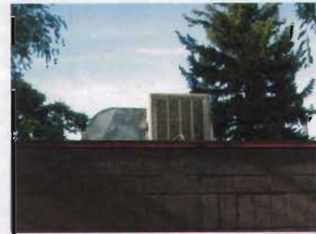
This roof mechanical system at 442 North 300 Street is set back so that it is not readily visible from the street.
