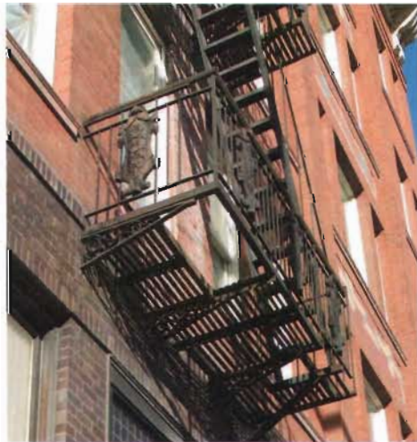
Proper fire escape placement at 379 South Main Street.
