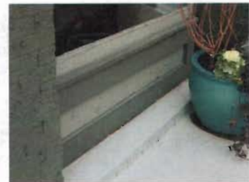
This rebuilt bulkhead at 361 North Center Street is a good example of in kind replacement.
