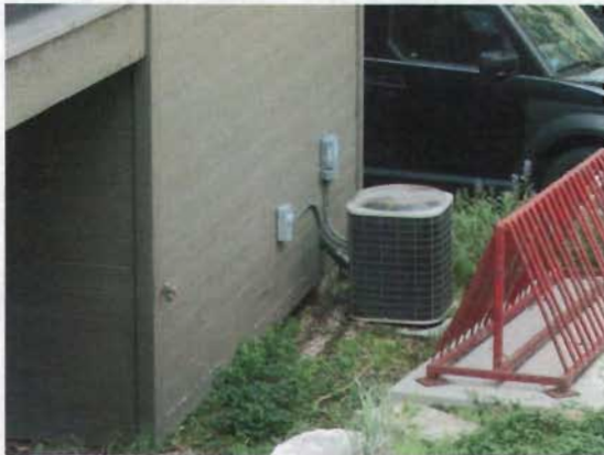
This HVAC system at 271 Center Street is situated in an inconspicuous area on the rear elevation.
