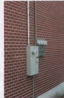
Meters at 39 North I Street are correctly placed on a non-primary elevation.
