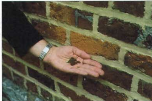
which leads to cracking and spalling.
