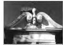
Elements such as window hoods, brackets and columns are often associated with particular styles and therefore their preservation is important.
