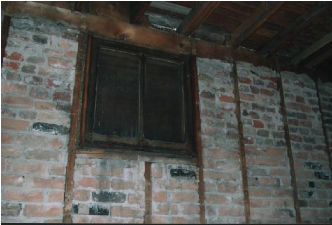
This window is where the chimney used to be--evidence that the missing chimney was not original.
