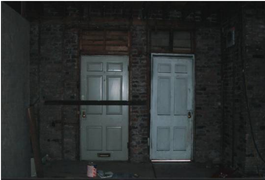
Partial sill to left of the left door shows that the second door was a later addition.
