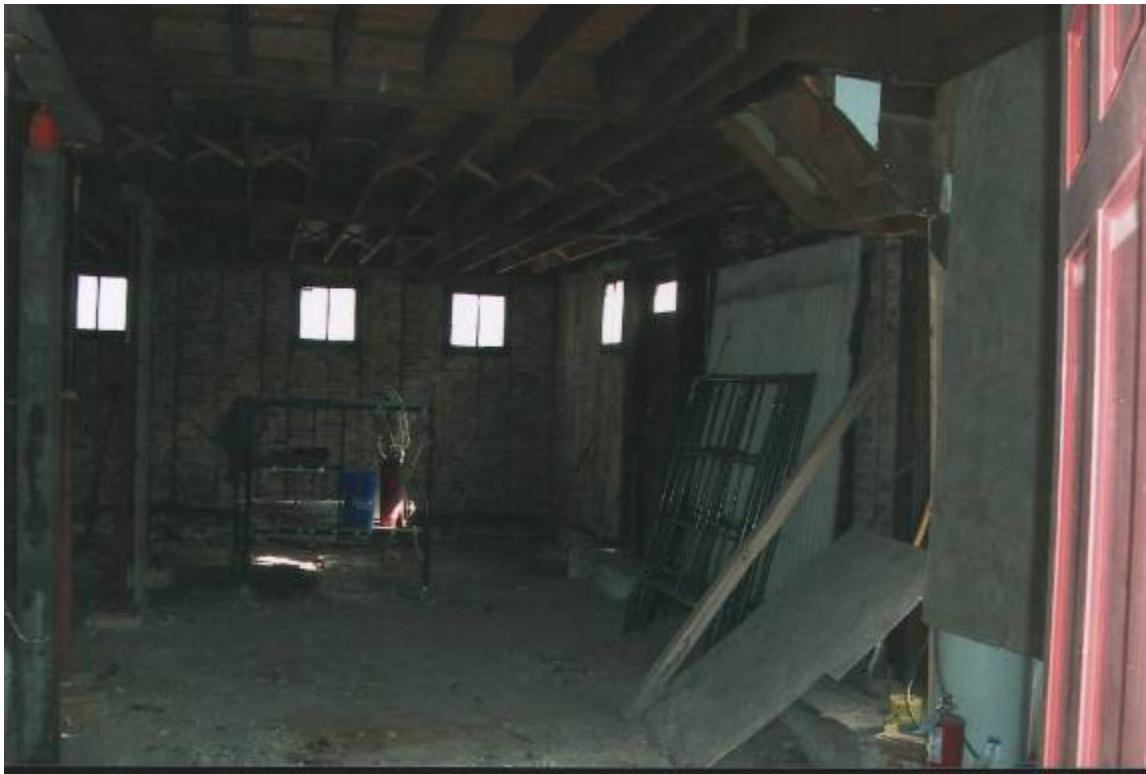
To the right is the sliding barn door which was removed prior to the 1970s documentation.
