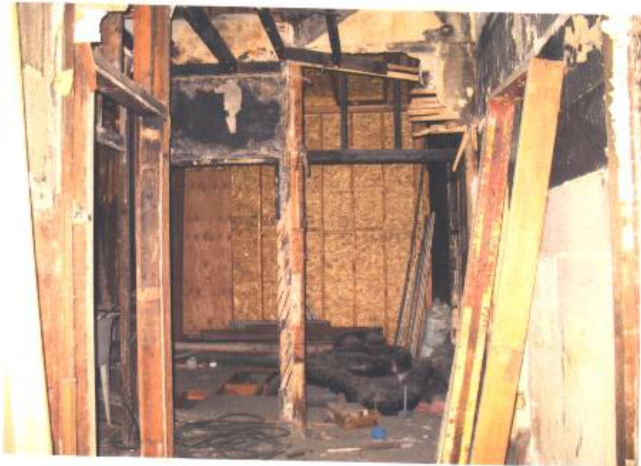
Fire and structural damage.
