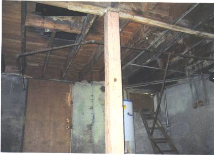
View of flooring system from basement. A hole in the floor can be seen. The hole was caused by a fire started by a transient. In the lower right hand corner shows placement of a ladder where transients and vandals accessed the home.
