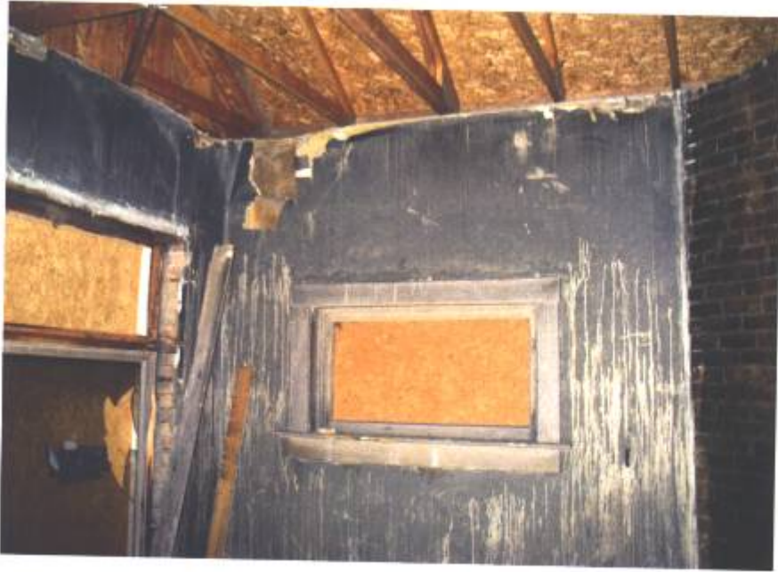
Water damaged walls.
