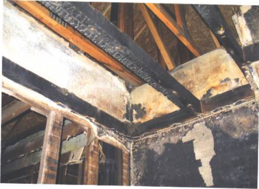
More fire damage.
