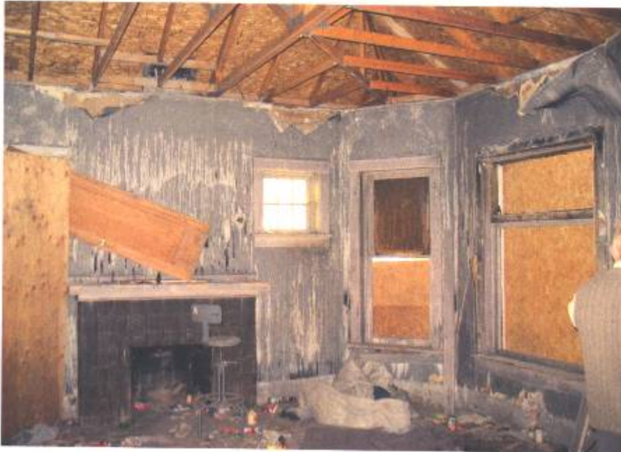
Walls show signs of water damage from fire.
