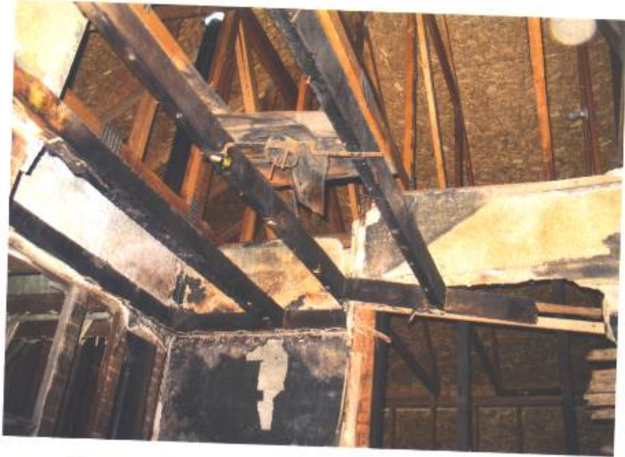
There was a fire in the back of the home. Picture shows damage.
