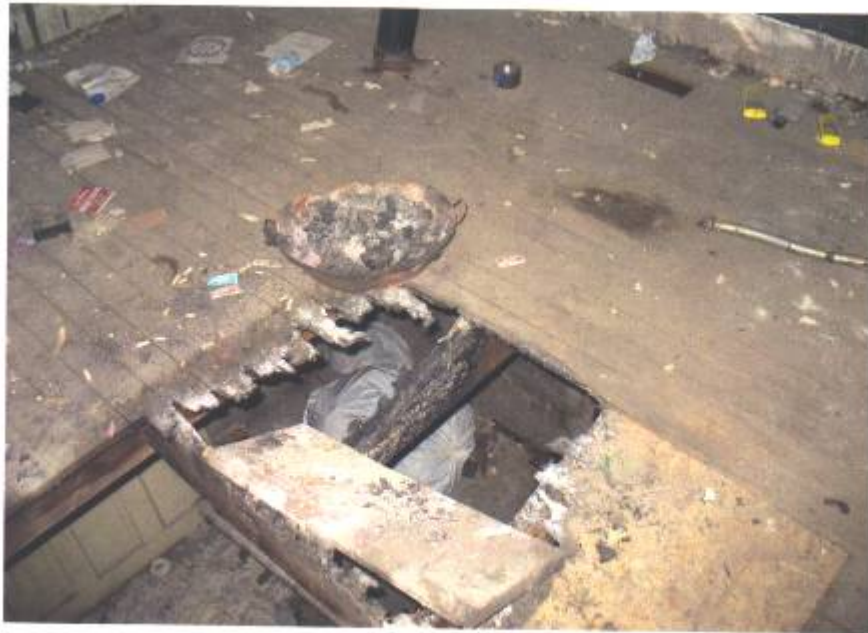
Top view of hole in the floor caused by a fire.
