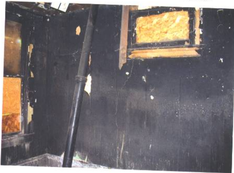
More fire damage.
