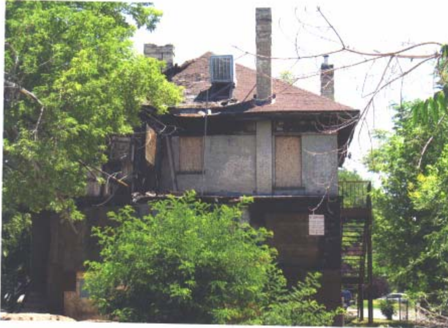
Rear of property. Evidence of unsound roof.
