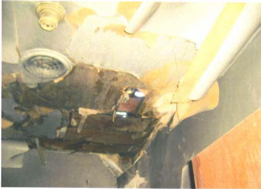
Roof in upstairs room showing water damage holes to the outside.
