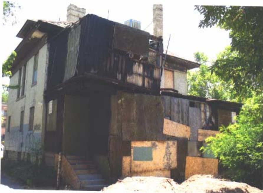
Rear of property showing burnt out rear addition
