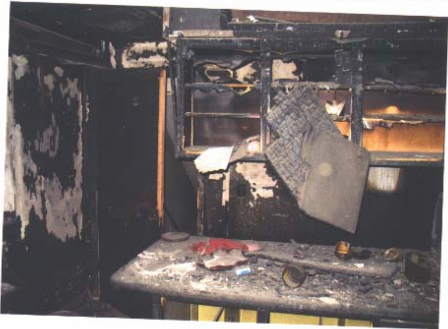
Fire damage to kitchen.
