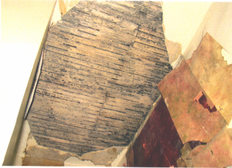
Fire and water damaged roof
