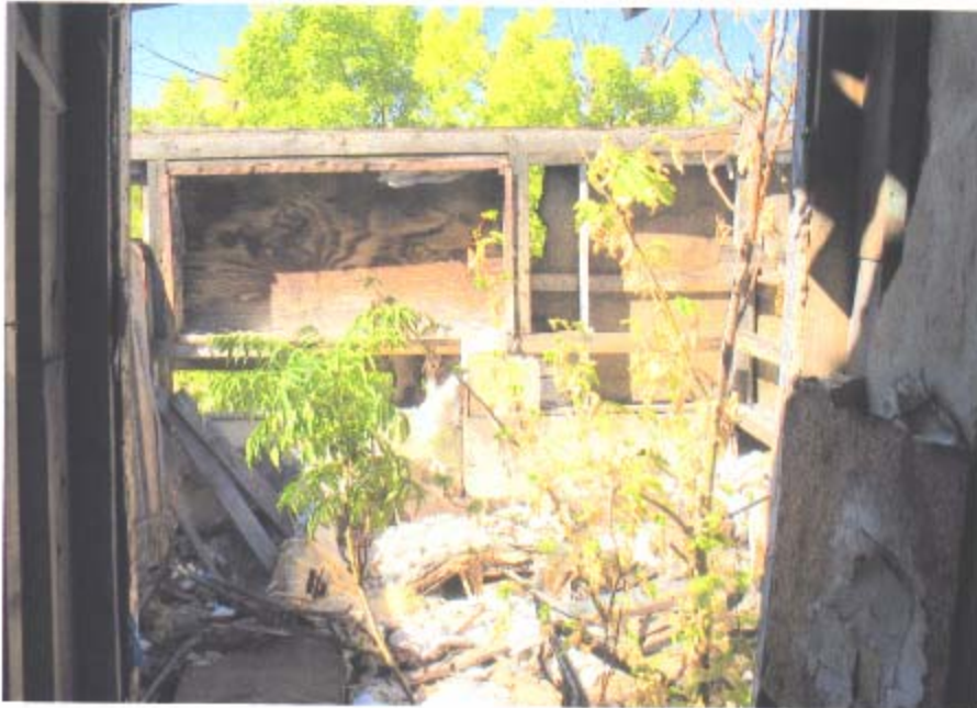
Upper floor of rear addition. Open to the elements with trees growing out of it.
