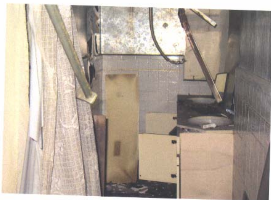
Main floor bathroom. This is the only bathroom in the home. It has been extensively vandalized.
