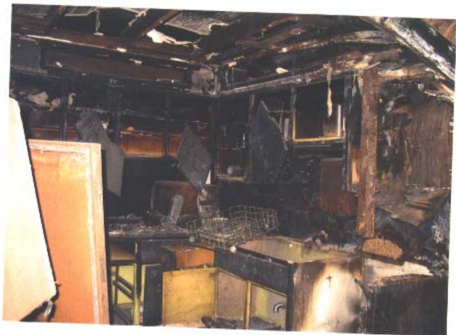
Fire damage to kitchen. This is the interior of the addition on the back of the home.
