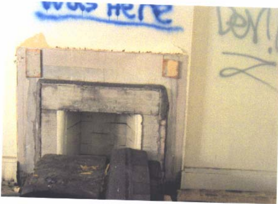
Front room fire place. The mantle and decorative tile has all been stolen.
