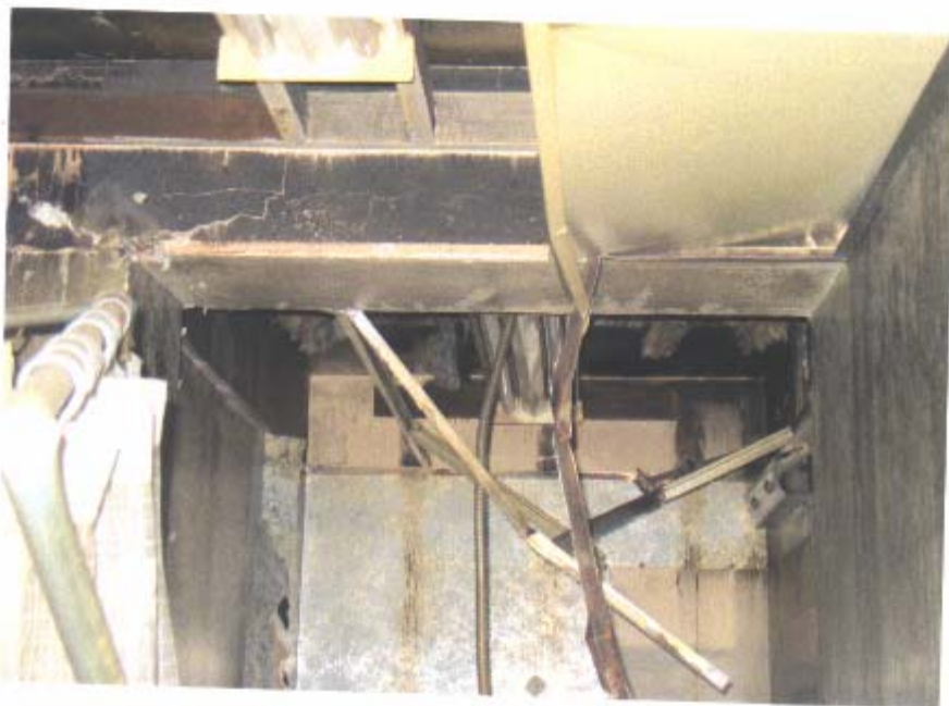
Main floor bathroom. This is the only bathroom in the home. It has been extensively vandalized.
