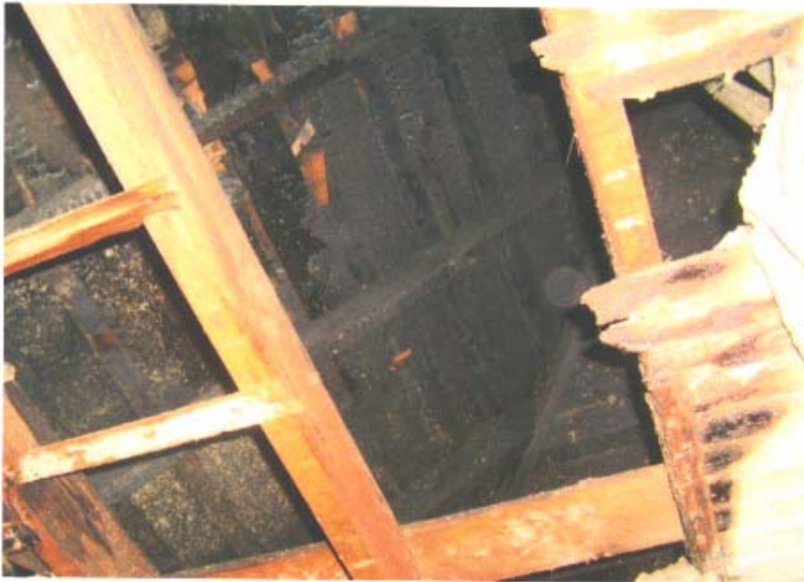
Fire damage to roof.
