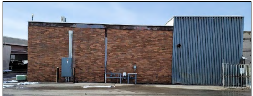
View of neighboring property to the west (Industrial Heat Treat) from the front of the property
