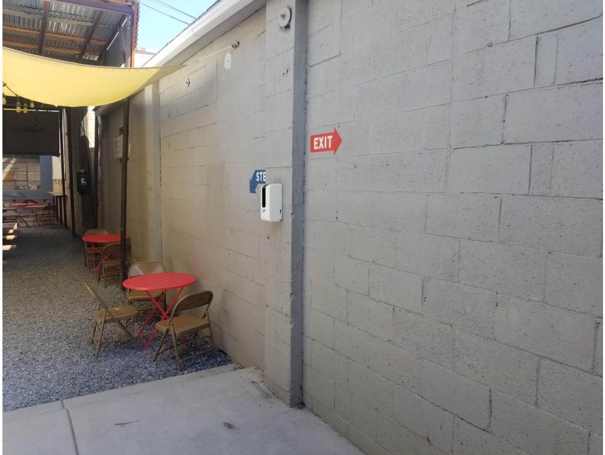
Photo 6: West wall of expansion building 778 S. 300W. from the existing outdoor patio area. This wall will be altered to accommodate overhead doors, man doors and windows to connect the new Tavern space. See the elevation drawings for more details.
