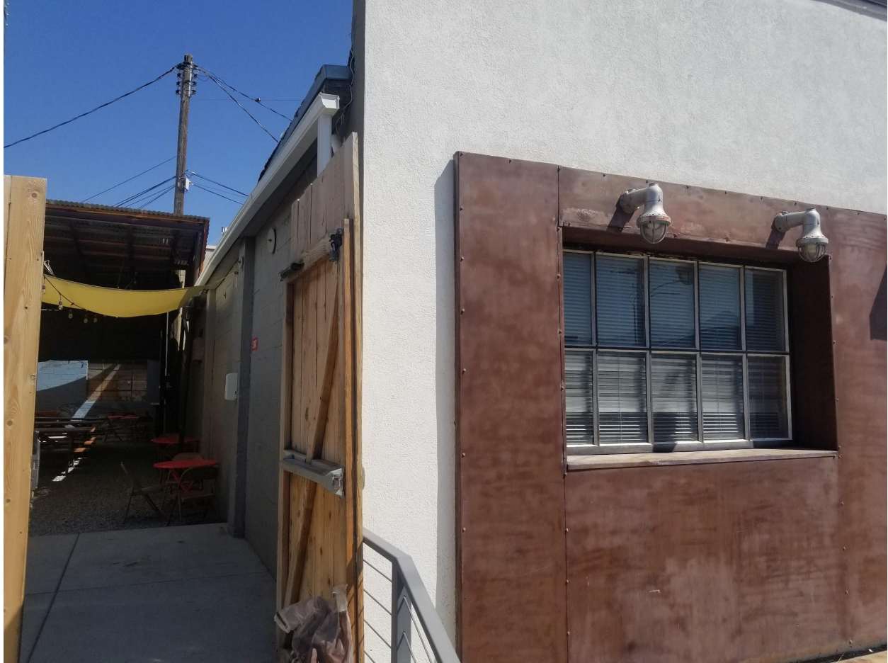
Photo 5: View from sidewalk into the existing west outdoor patio gate with the expansion building shown on the right.
